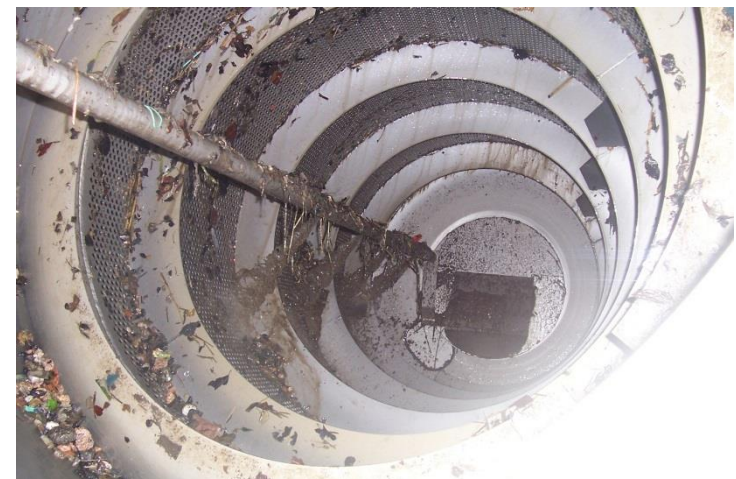
View into a Wash Drum
