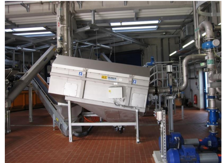
Wash Drum on WWTP Oldenburg
